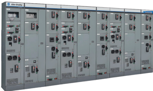
Control panel protection
