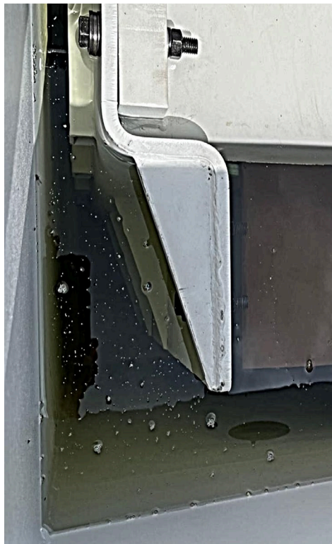
Figure 4: Dissolved Gasses Manifesting in the Insulating Fluid of a Distribution Transformer
